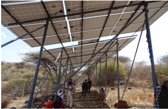
Bangole Solarized system in Marsabit
